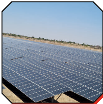
WORLD'S LARGEST SOLAR PARK (5000 MW)
